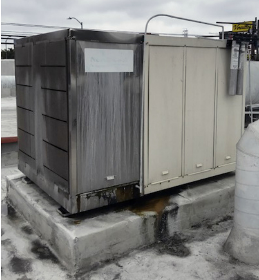
Versailles rooftop swamp cooler.
