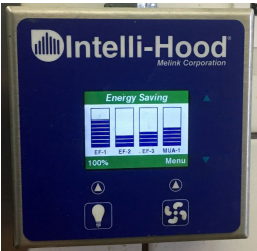
DCKV control interface showing individual exhaust and makeup air fan speeds.
