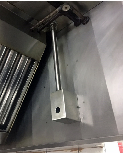
DCKV in-hood air opacity sensor.
