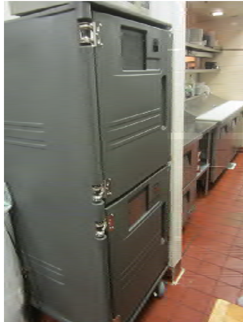
Figure 44: Plaza Suites Replacement Holding Cabinet
