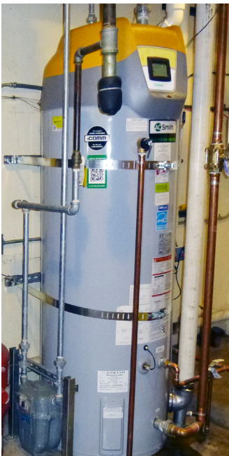
Replacement Condensing Water Heater
