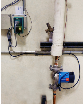
ECM Circulator and recirculation pump controller
