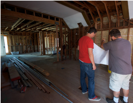
Mark (left) and Matt Greco surveying the future kitchen space of SaltCraft.
